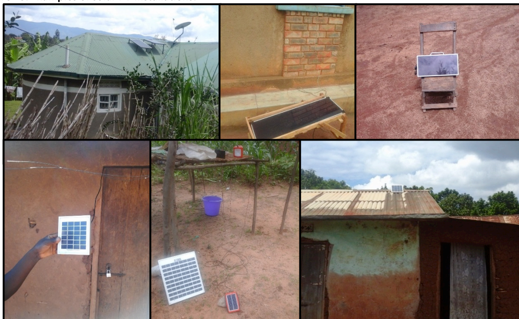
Figure 13. Examples of solar PV installations.
